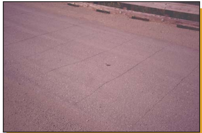
Figure 3—Cracking over panel joints on the Watchtower Creek Bridge at the Bitterroot National Forest, MT, in 2000.
