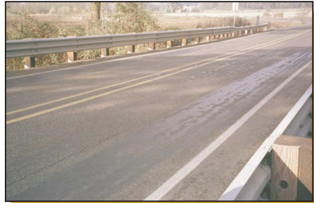
Figure 21—Alternating longitudinal deck panels treated with penta and copper naphthenate on a bridge in Washington County, OR.
