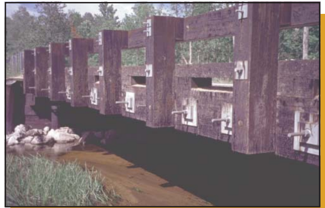
Figure 14a—The Cruzen Bridge in Alcona County, MI, was made from timbers that had not been cleaned properly after being treated with preservative.
