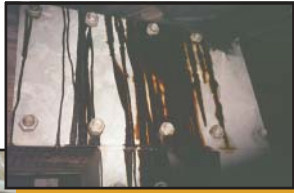
Figure 20a—Cooled asphalt dripping from the underside of the LaChance Bridge in Michigan.
