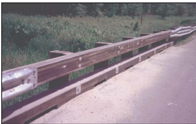
Figure 13b—Proper cleaning prevented creosote-treated timbers from bleeding through the asphalt pavement on the Barlow Bridge.
