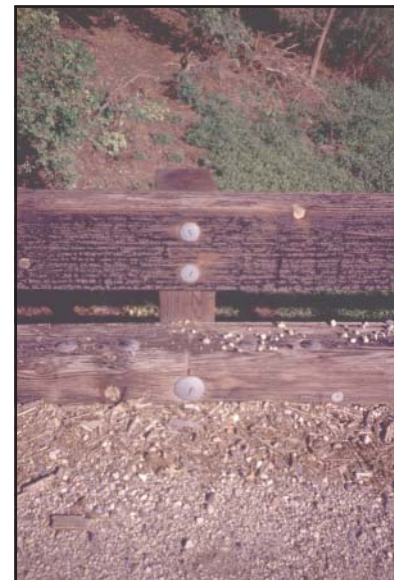
Figure 14b—Creosote-treated timbers on the Cruzen Bridge were not cleaned after treatment. Creosote is leaching from the timbers.
