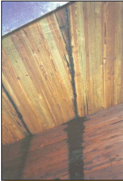
Figure 22—Rubberized asphalt dripping from paving membranes on the Rogue River Bridge near Medford, OR.
