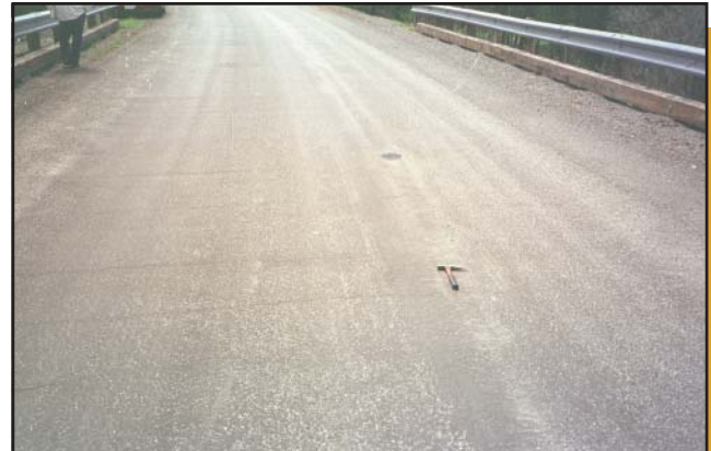
Figure 6—Bridge across Wolf Creek near Libby, MT, showing minimal cracking.
