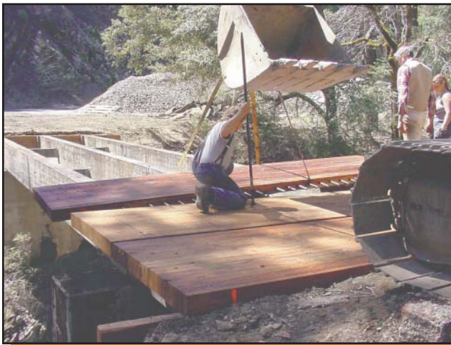
Figure 7—Dowel-interconnected, transverse glued-laminated deck panels on the Mill Creek Bridge near Medford, OR.
