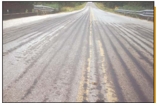
Figure 16—Asphalt bleeding directly over creosote concentrations on the Cruzen Bridge in Alcona County, MI.
