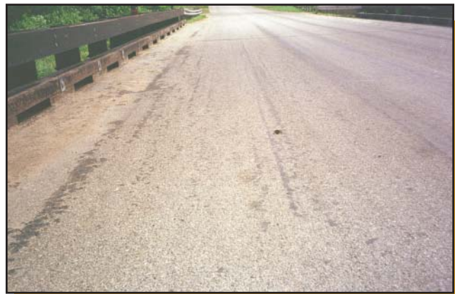
Figure 15—The Cameron Bridge in Crawford County, MI, had asphalt bleeding over glued-laminated webs.
