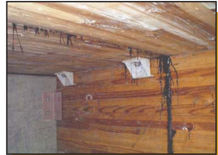
Figure 24a—Rubberized asphalt dripping from the underside of the Shady Cove Bridge.
