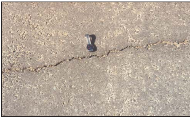
Figure 2—Cracking over panel joints on the Watchtower Creek Bridge at the Bitterroot National Forest, MT, in 1989.
