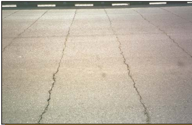
Figure 11—The pavement cracked about 1 year after construction of the Standish Avenue Bridge in Petoskey, MI.
