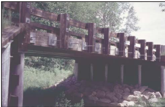
Figure 13a—The Barlow Bridge in Alcona County, MI, was made from timbers that were cleaned properly after being treated with preservative.
