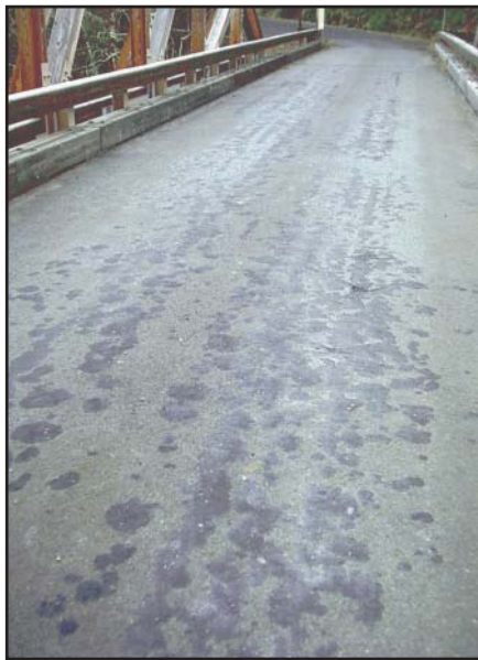
Figure 23—Asphalt leaching to the pavement surface of Shady Cove Bridge near Eugene, OR.
