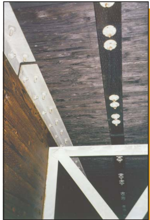
Figure 8—Deck stiffener beams installed under transverse glued-laminated deck panels on the Lighthouse Bridge near Port Angeles, WA.
